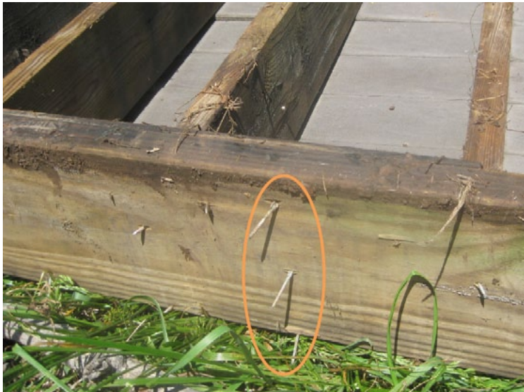
Figure 1. Close-up of deck ledger that was connected to a structure with nails only. When lightly loaded by occupants, the deck shifted laterally, pulling the nails out of the supporting structure.
