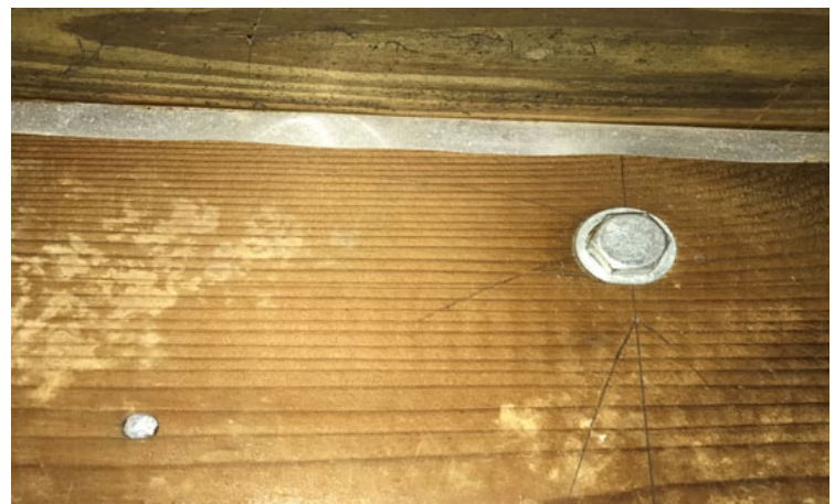
Figure 2. Section of a deck ledger with a nail head and ½” diameter lag screw installed.
